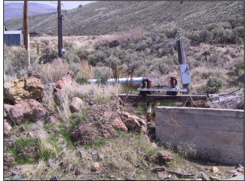
Figure 30. Irrigation pump facility.
